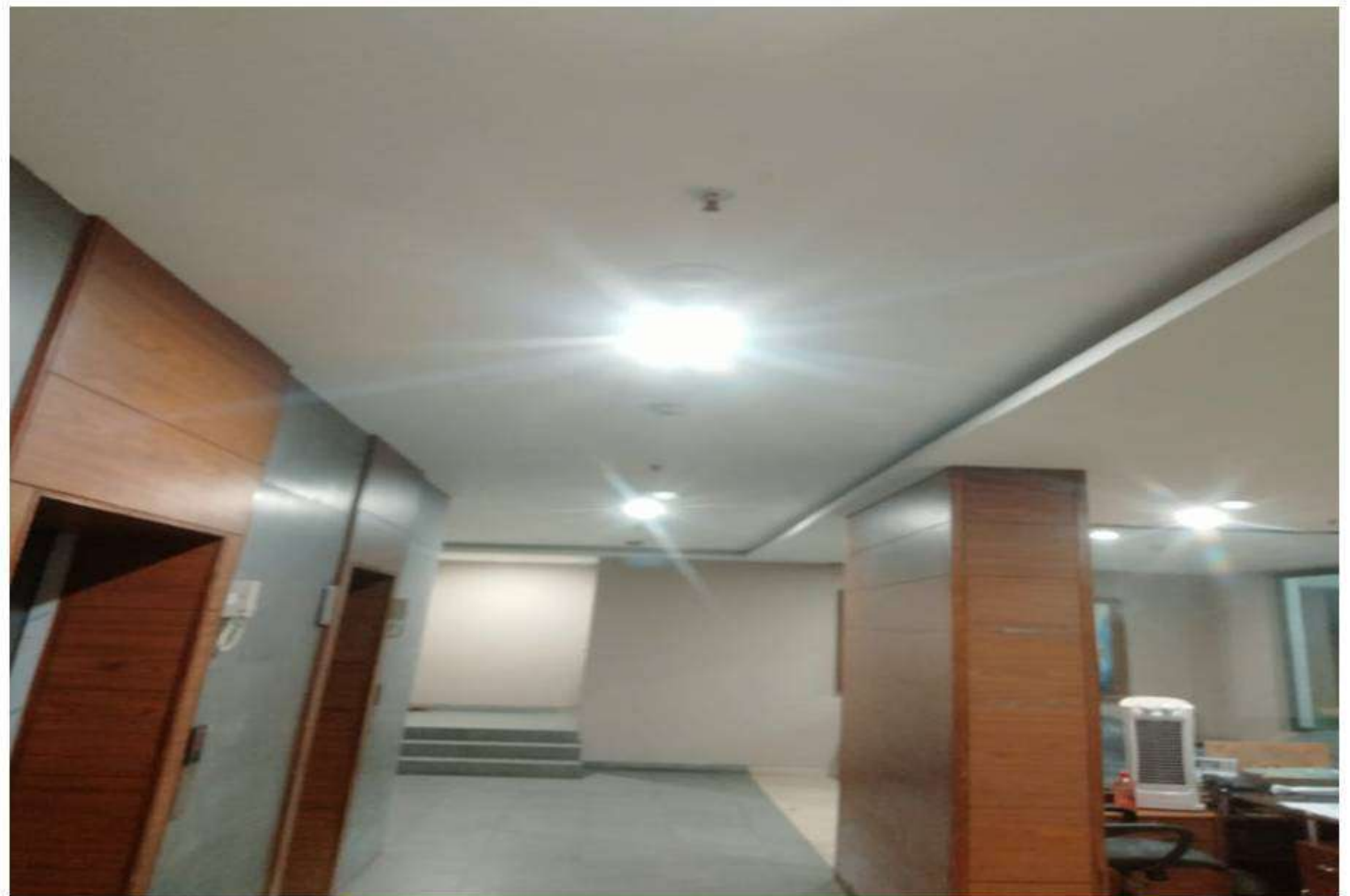
Fire protection and detection in common area
